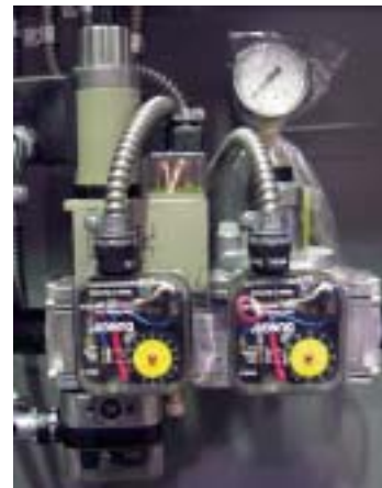
Figure 9 - Dungs high/low gas valve helps prevent oven fires and speeds processing.
